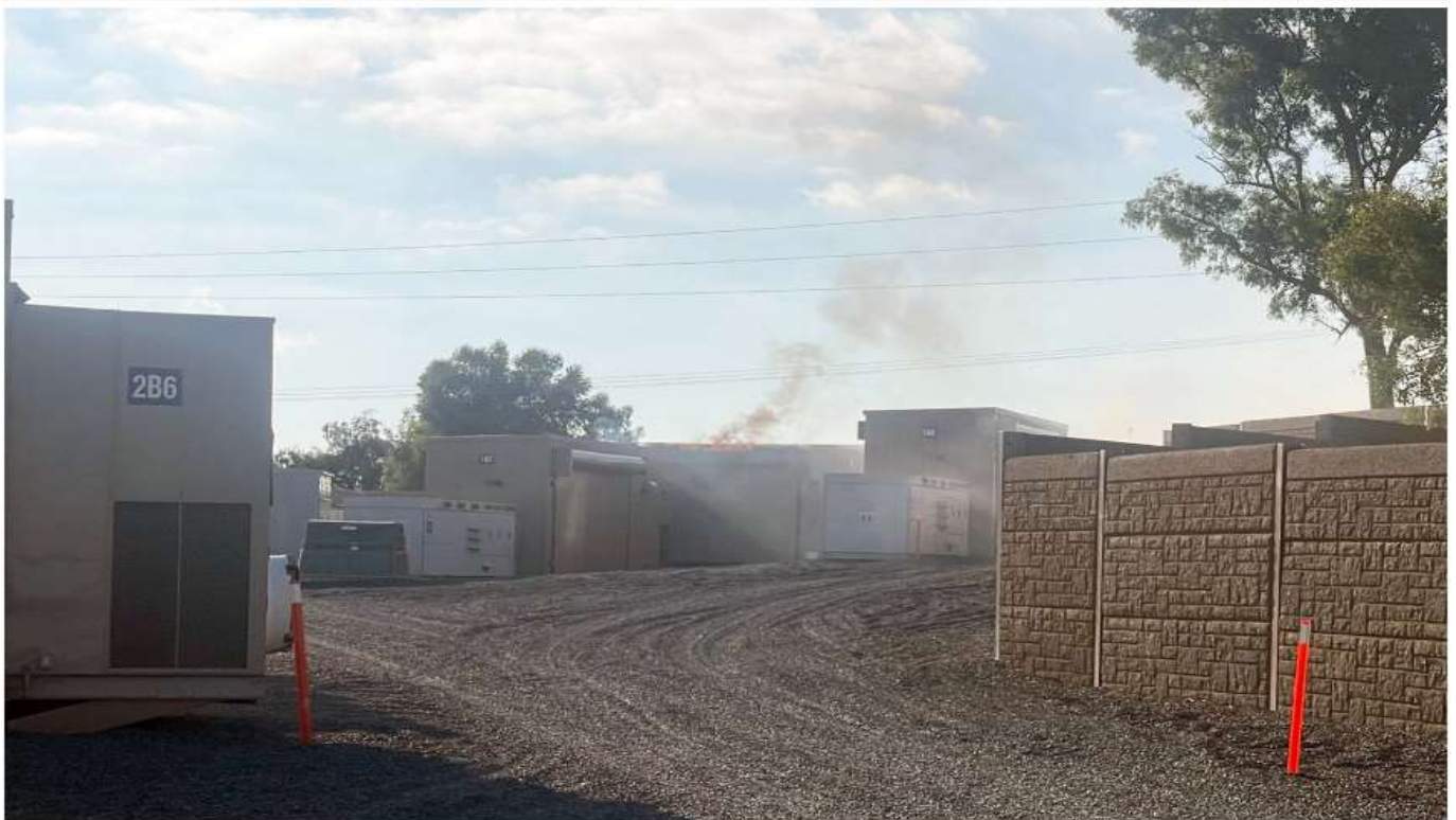
Fig. 2 Battery energy storage system fire incident in Terra-Gen at Sen Diego
