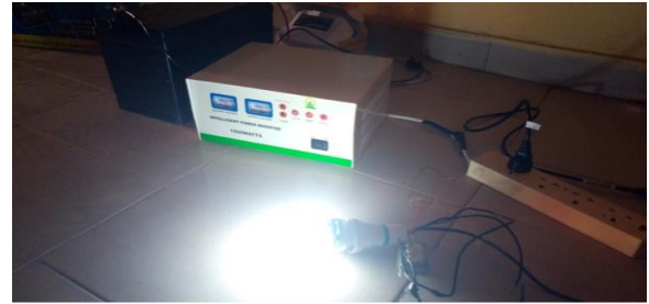
Figure 13: Testing the Inverter and Battery with Loads.
